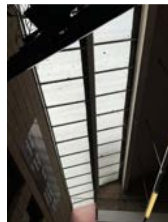
FIGURE 9 INTERNAL VIEW OF LIGHTING PANELS AT HIGHFIELDS UPPER
